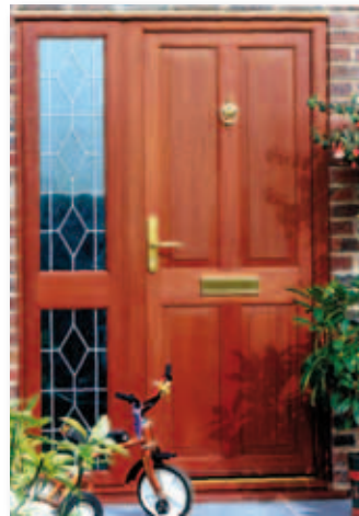
Front door with raised and fielded panels and a full height leaded sidelight. The sidelight midrail aligns with this door but the head and kick rails do not
