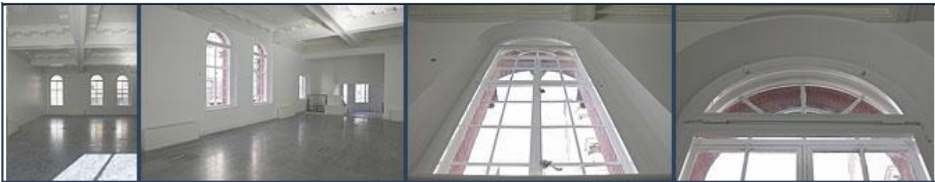
Primary Windows with Semi-Circular Heads - Secondary Glazing Replicates Design & Secondary Glazed Semi-Circle Hinges In using Bespoke Hinge & Turnbuckle System Design & Produced Specially for this Contract
